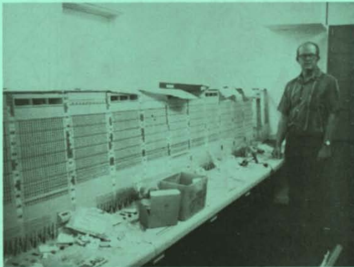
Chuck Deemer, Western Electric leadman for our installation, works on the new switchboard.
